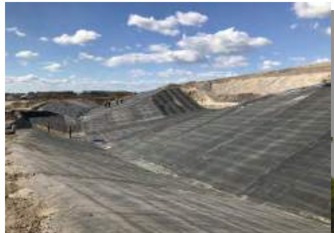
Drainase Air Hujan, Kogan Creek Site - Australia
